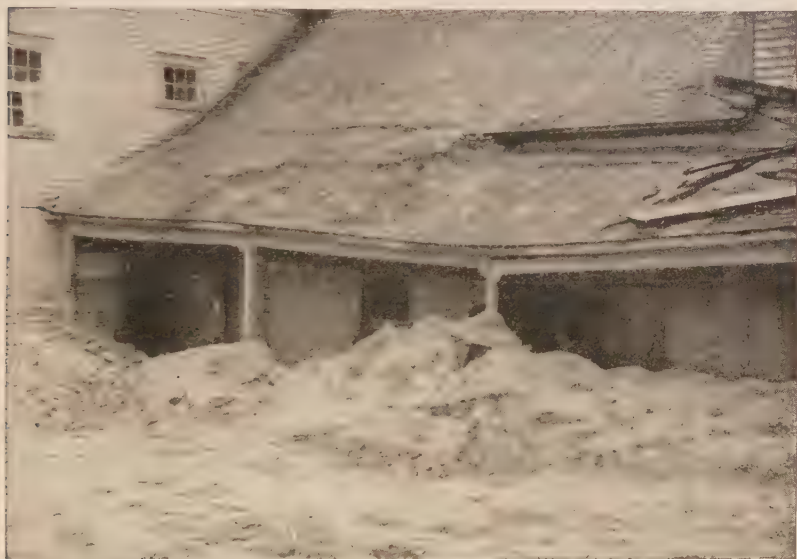
FIG. 298. — A roof collapsed by the weight of ash from Katmai, Alaska, one hundred miles distant. The drift in front of the porch is volcanic ash. ( National Geographic Magazine .)
